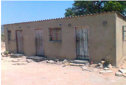
Plate 4. 2: Sub-standard building structures at Mutawatawa growth point
