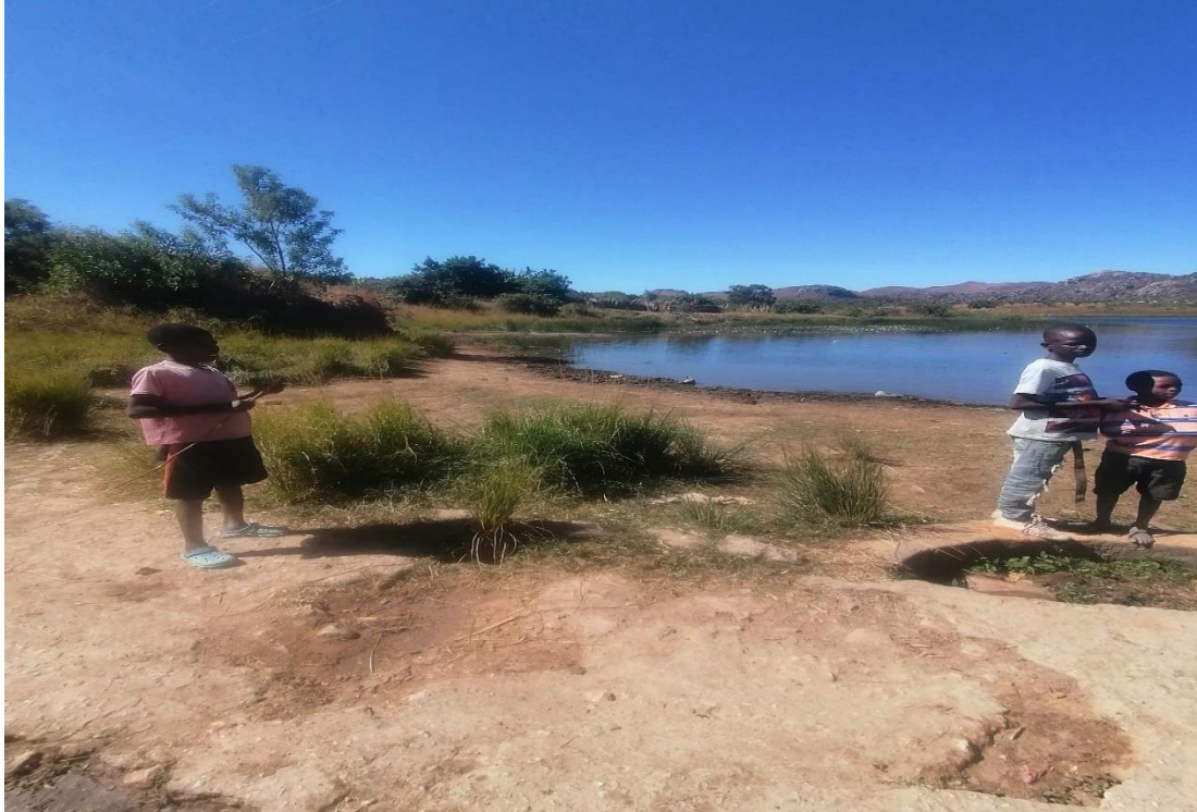
Figure 5: image of heavily silted spillway and juvenile fishermen at Syalima dam
