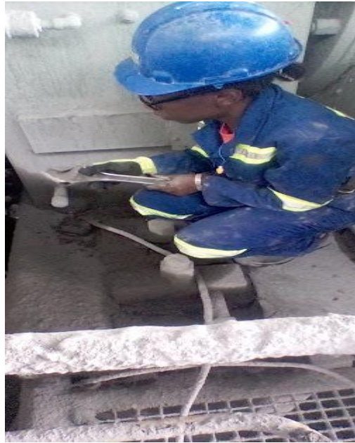
Figure 1.1 Trouble shooting the water sensor at Tank 23
