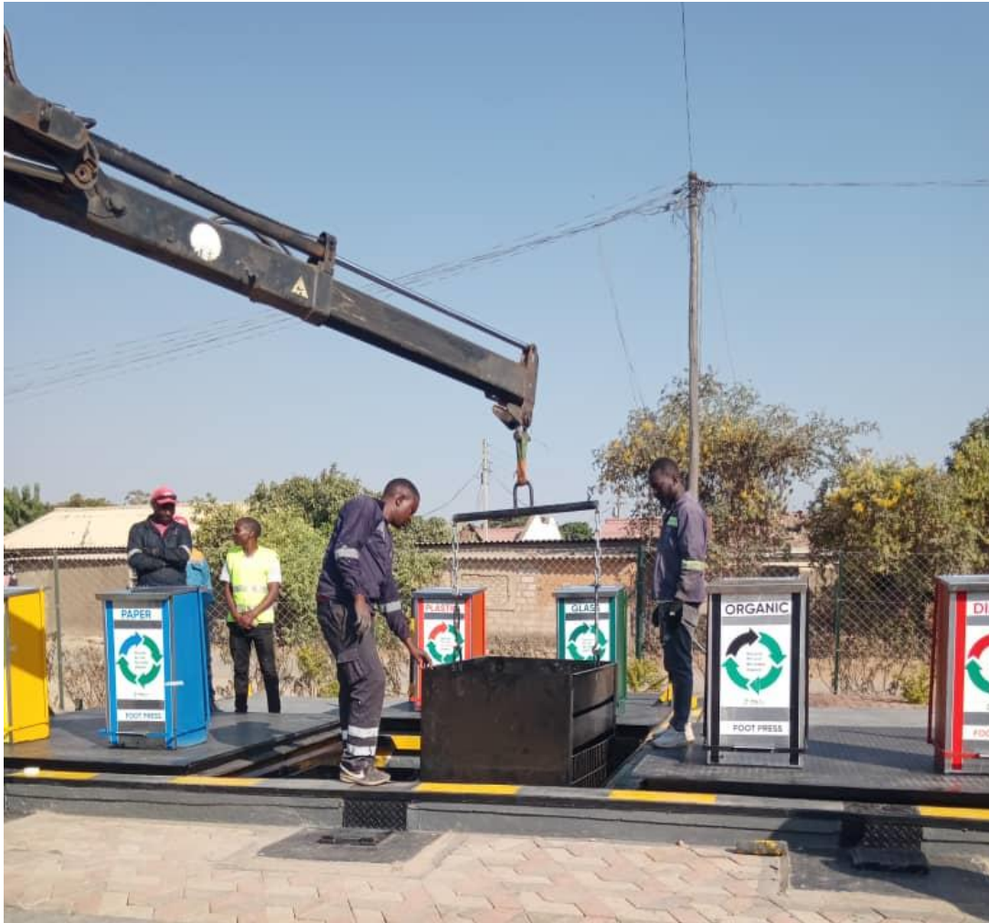
FIG 4.5 shows the underground bins at the Mavambo Shopping area in Ruwa
