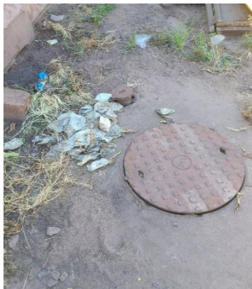
Figure 4.24 shows a drainage blockage to mask waste.
