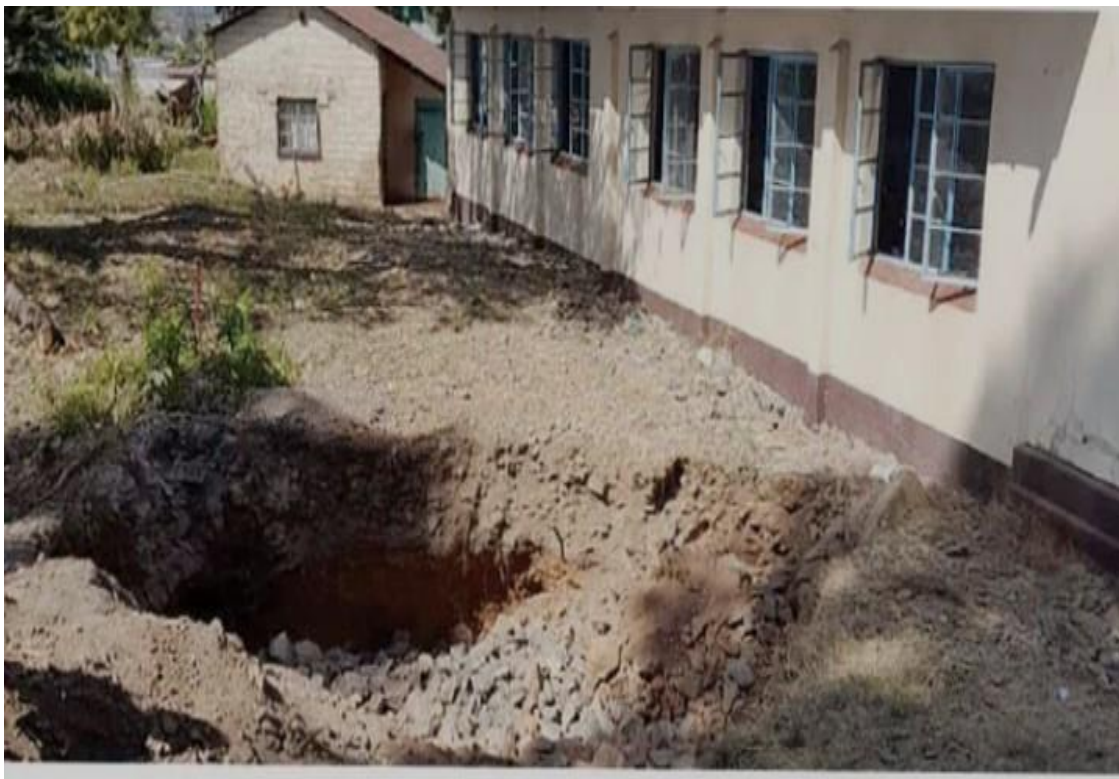
Figure1: Figure showing the type pits dug at Globe and Phoenix Primary School and at other areas around Globe and phoenix.
